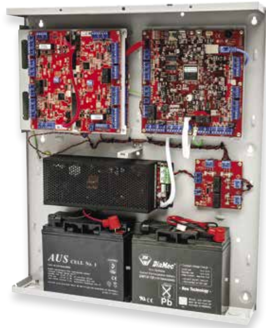
ABOVE: IAC shown in 8 Door / 10 Reader configuration. (IAC with UniBus 2 Door / 2 Reader expansion devices connected). Housed in the WideBody enclosure with hinge plate, 8Amp PSU, Fire Door override relay card and 2x 17Ah batteries
